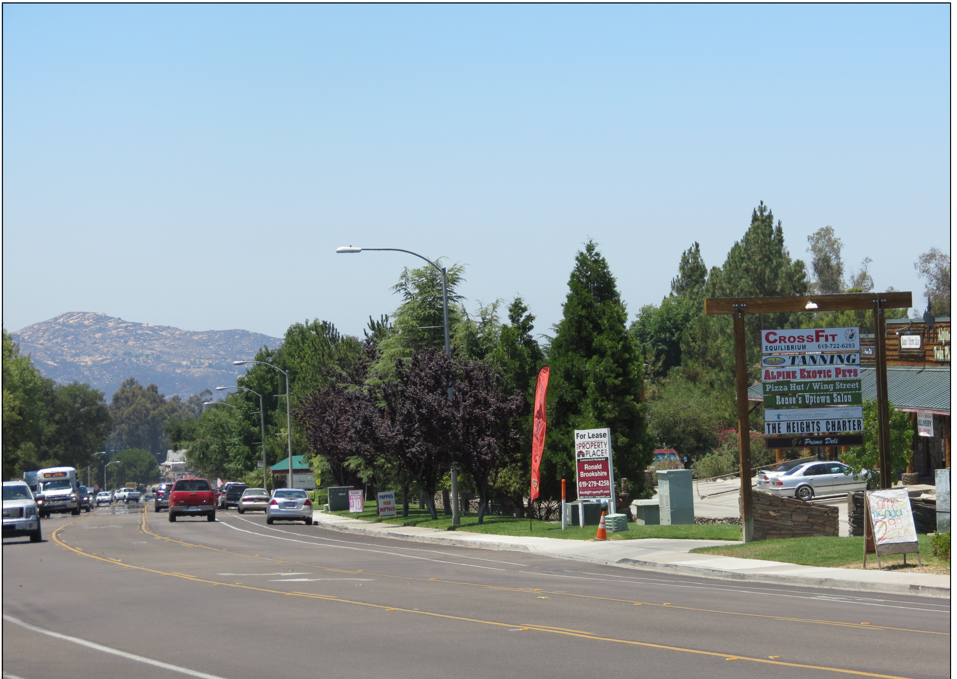
ALPINE BOULEVARD'S NEW LOOK AFTER THE SUNRISE POWERLINK TOOK OUT POWER POLES AND INSTALLED UNDERGROUND UTILITIES—2013
